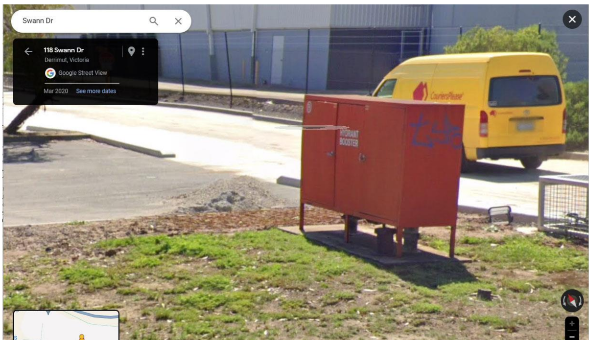
Hydrant booster at front of property
